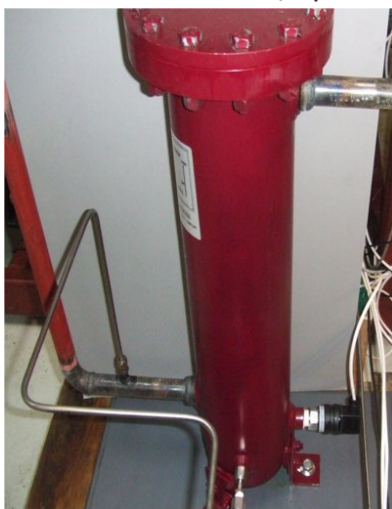
HBSO Oil Switch on a Filter/Separator
