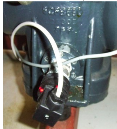
HBSO Oil Switch on a Compressor
